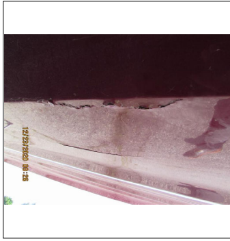
Longitudinal Fractures Port side Centerline
