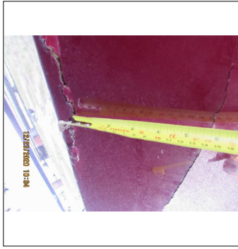
Distance between Longitudinal Fractures
