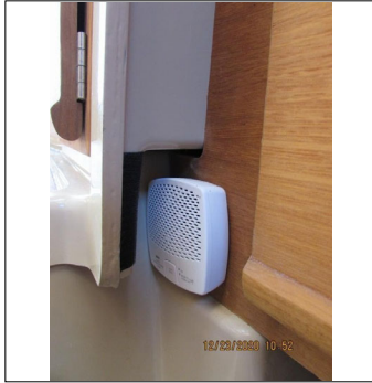
CO Detector Improperly Installed
