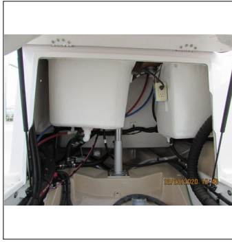
125VAC Receptacle Installed in Gasoline Fuel Space
